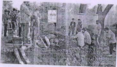
Waste water management project
