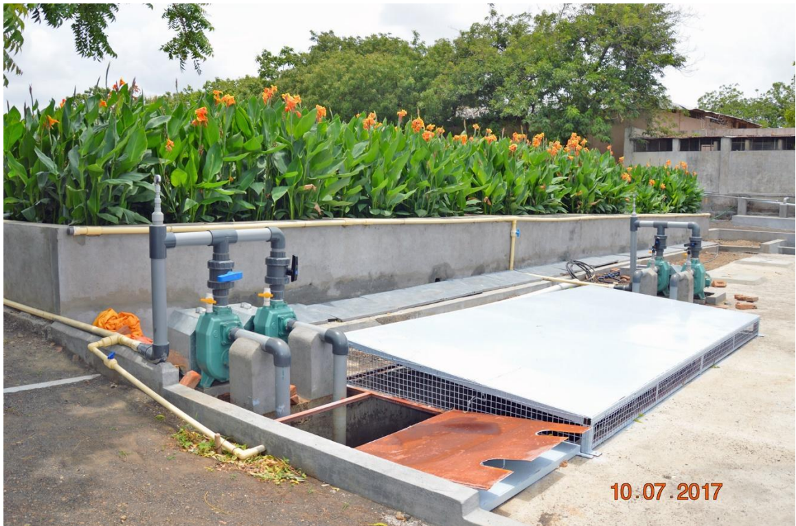
Waste Water Plant
