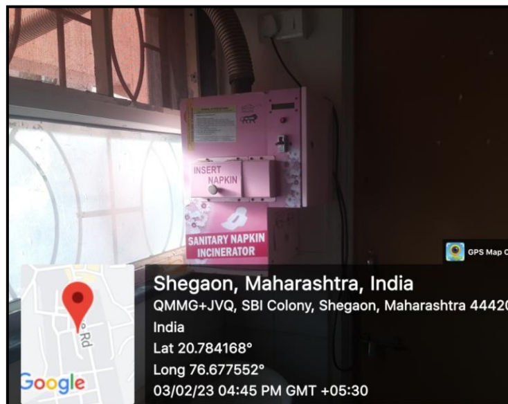
Sanitary waste incinerator
