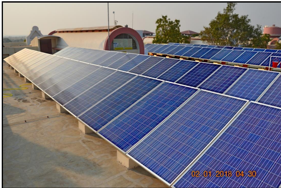
Photograph of Solar PV Plant:
