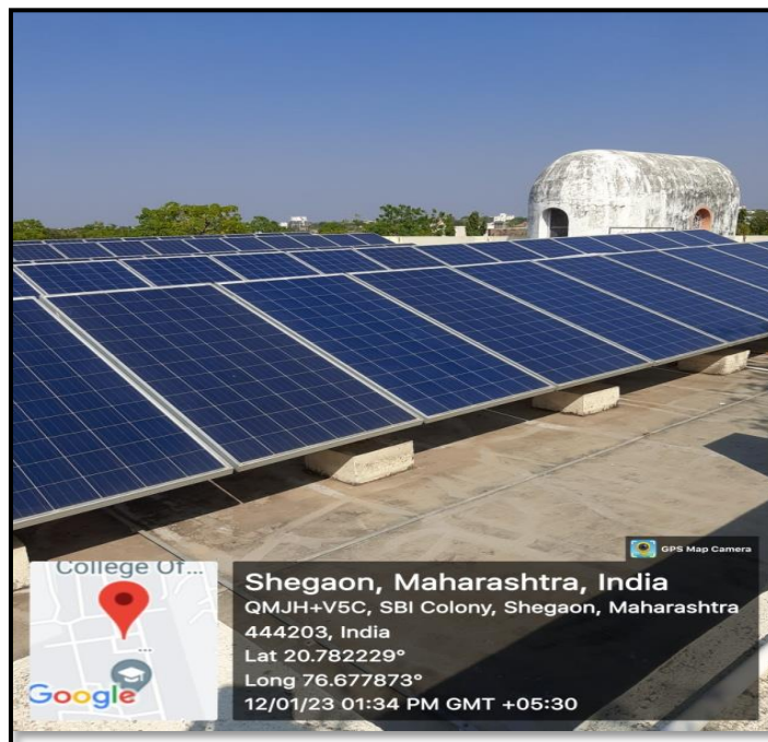
Photograph of Roof Top Solar PV Plant:
