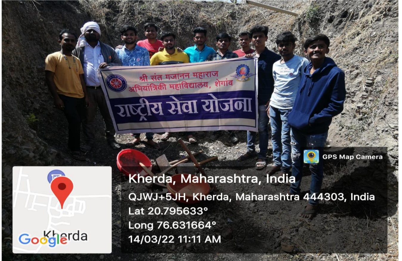
The digging of pits aimed to create storage reservoirs for rainwater 14th March 2022
