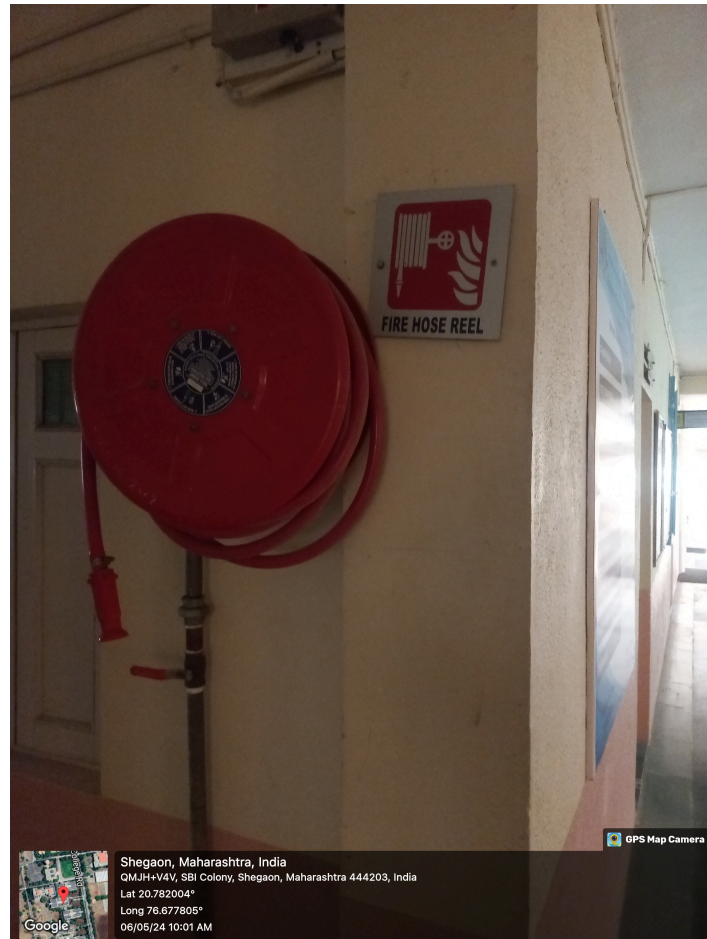
Fire House Reel
